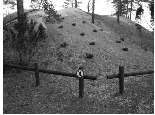
Fig. 3. The dune slope facing the campsite was covered with geotextile and mountain pines were planted on the slope
